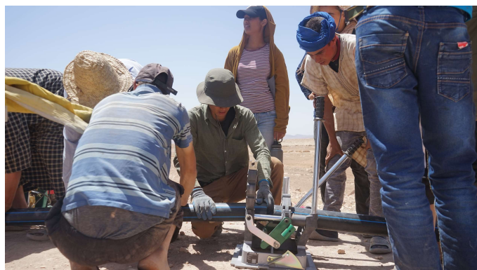
Figure 7: Team members and community members working together to fuse two lengths of pipe
